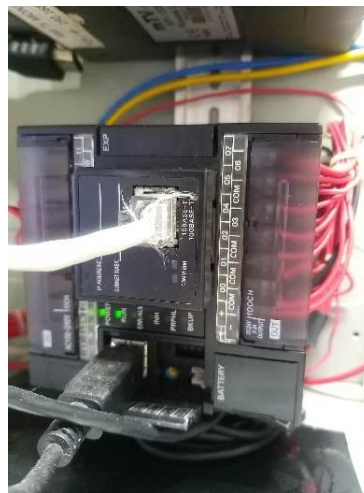
Figure 6. Indicator CP1W is not connected between PLC and HMI
