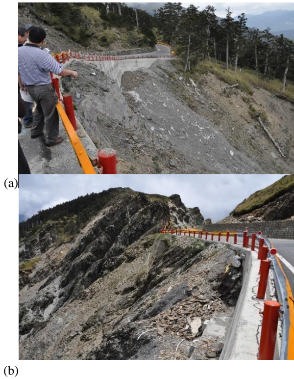
Figure 1. Photos about the (a)northern part and (b)southern part of the downhill slope at Kenanguan section. Multiple measures such as piles, retaining wall with anchors have been applied to mitigate the roadbed subsidence problem.
