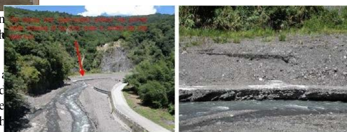
Figure 7 Honghsiang mixing land improvement engineering method used to protect against slided land
