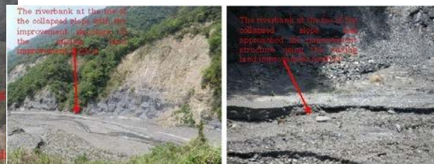
Figure 6 Hewang mixing land improvement engineering method used to protect against slided land
