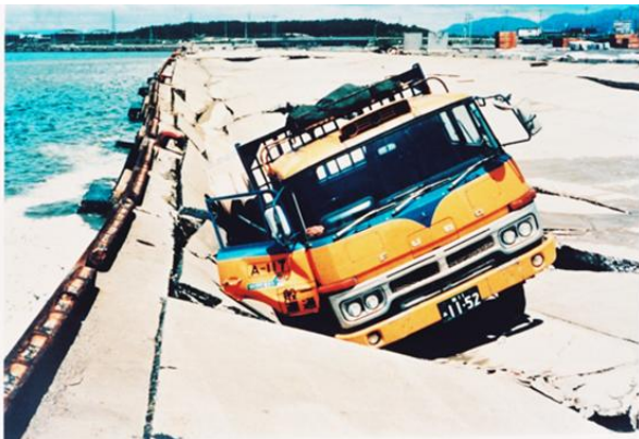
Figure 5 Damage to a sheet pile quay wall due to liquefaction of backfill soil at Akita Port during 1983 Nihonkai-chubu earthquake (after Akita Prefecture)
