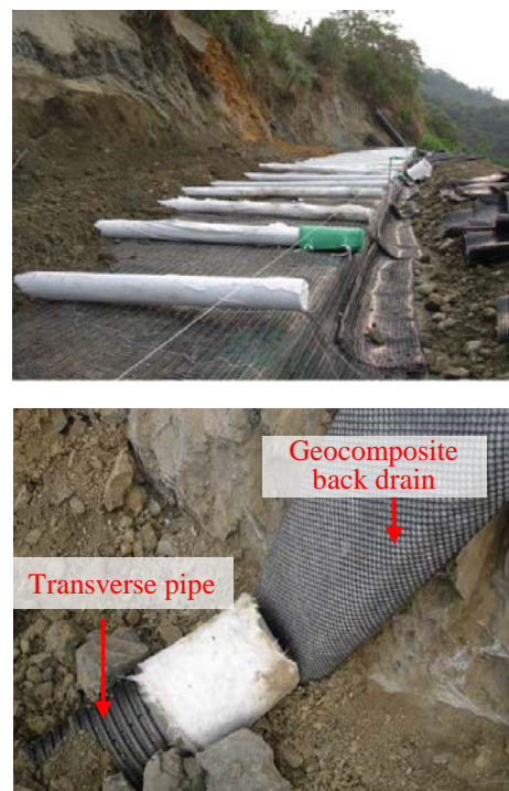
Figure 4. Drainage installations: (a) transverse drains; (b) back drain and transverse drain connection joint
