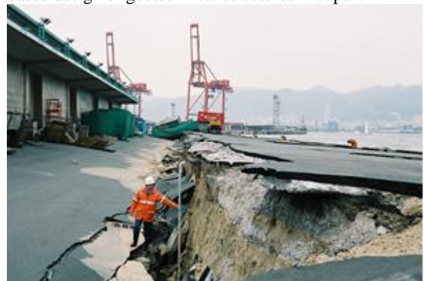
Figure 6 Damage to a caisson quay wall at Kobe Port, Japan, during the 1995 Hyogoken Nambu earthquake
