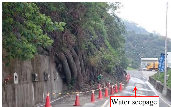
Figure 6. Close view of failed slope at the toe
