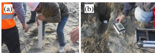
Figure 4 Borehole drilling and vibrometer embedding before the tests: (a) borehole drilling; (b) vibrometer embedding
