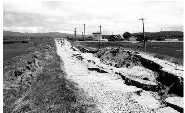
Figure 16 Damage to a dike at the Shiribeshi-toshibetsu river, Hokkaido, Japan, during 1993 Hokkaido-Nansei-oki earthquake
