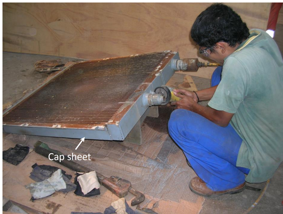
Fig.3. Cutting off the failed after-cooler around the leak location for sample preparation
