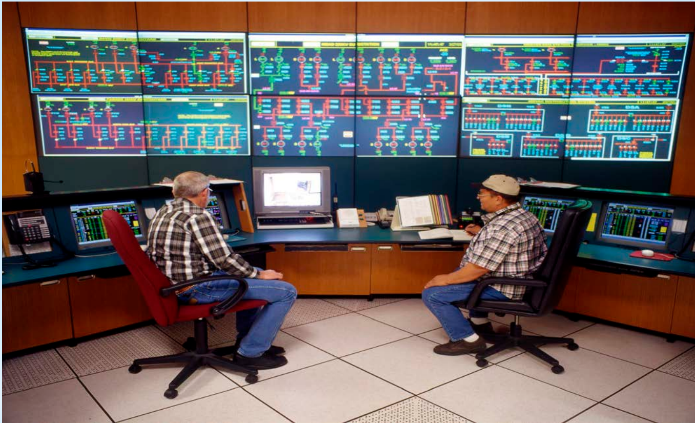
Ruang Kontrol Digital Hoover Dam Amerika
