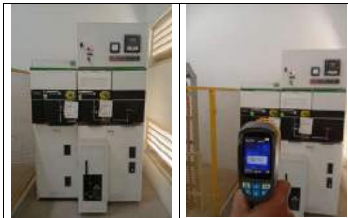
kondisi Existing panel PUTM
