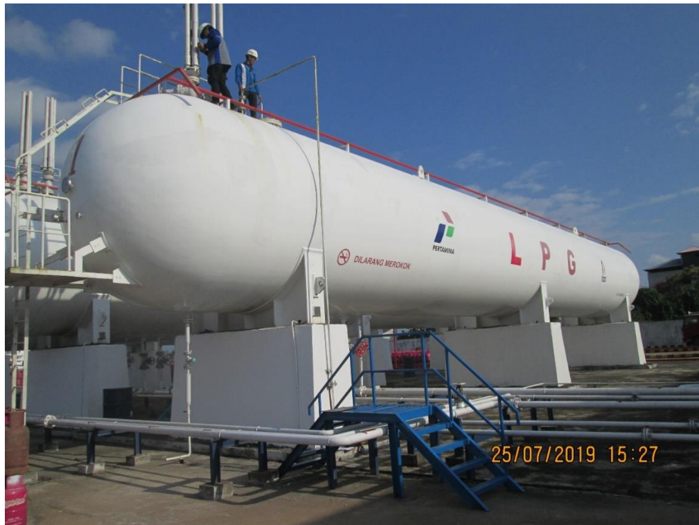
Gambar 2. 3 LPG Storage Tank
