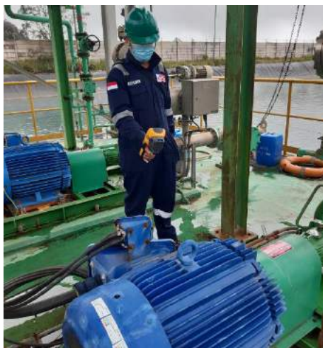
Gambar 2.14 Re-injection pump di PLTP Patuha Unit 1
