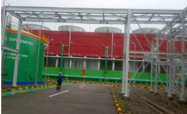
Gambar 2.12 Cooling tower PLTP Patuha Unit 1
