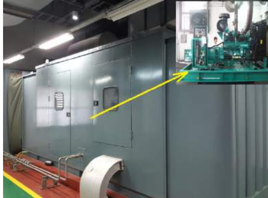
Gambar 2.15. Emergency Diesel Generator (EDG) di PLTP Patuha Unit-1
