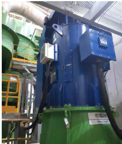
Gambar 2.13 Hot Well Pump (HWP) PLTP Patuha Unit-1
