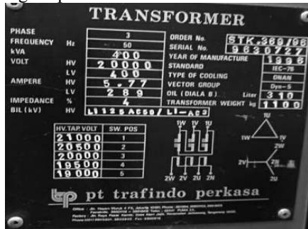
Gambar 12. Name Plate Transformator.
