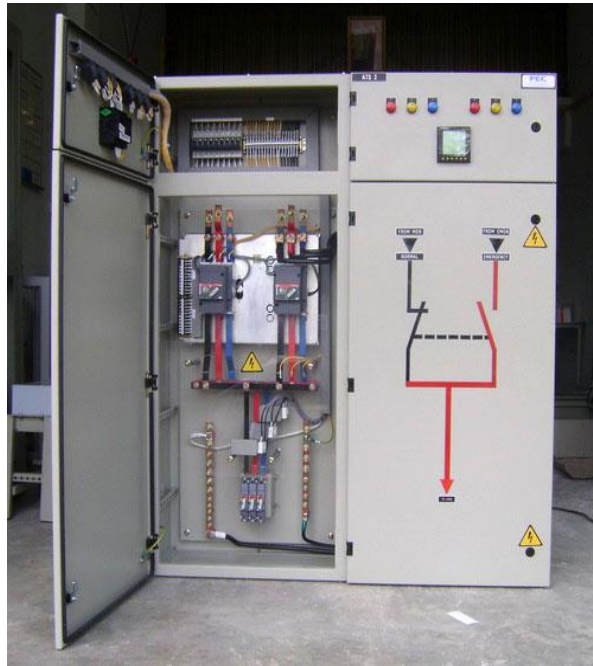
Panel Automatic Transfer Switch (ATS)
