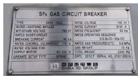
Gambar 10. Nameplate Circuit Breaker
